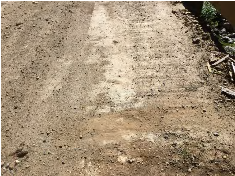
Damage noted to deck due to track equipment
