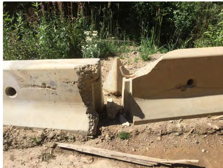
Damage to downstream left bank approach barriers
